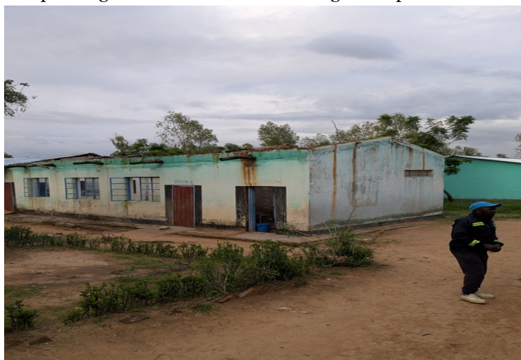
Effect of a storm: roof of a classroom of a visited primary school in Hurungwe blown off
